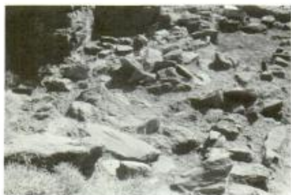
a. Fallen stones, from southwest
