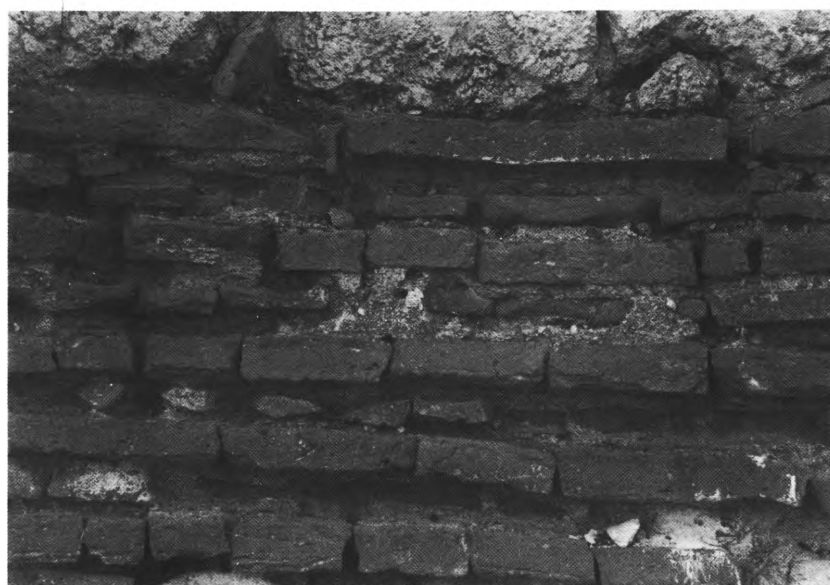
a) Pherrai, Kosmosoteira. South façade, «recessed brick» construction, b) Didymoteichon, Ag. Aikaterini. East façade, «brick filled mortar joints» construction.
